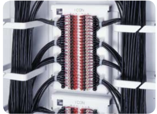
QCP II Termination Block (I-24A)
