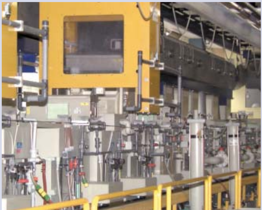
Partial view of the SUCOPLATE plating line
