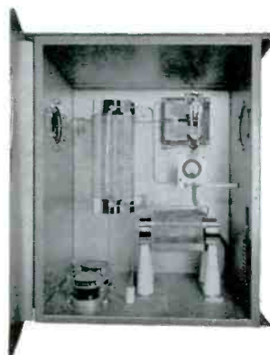
Line Terminating Unit MI-7485 enclosure. Open
