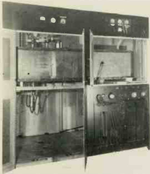
General View of Television Transmitter Using A-2027 Tetrode
