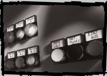
Labeling of push-buttons and signal lamps
